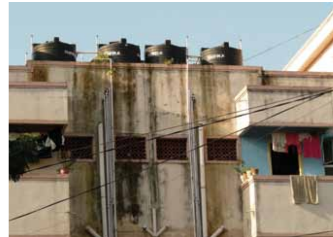
Figure 6: Urban Rainwater Tanks.
